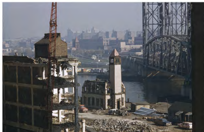
Industrial Decay / Demolition
